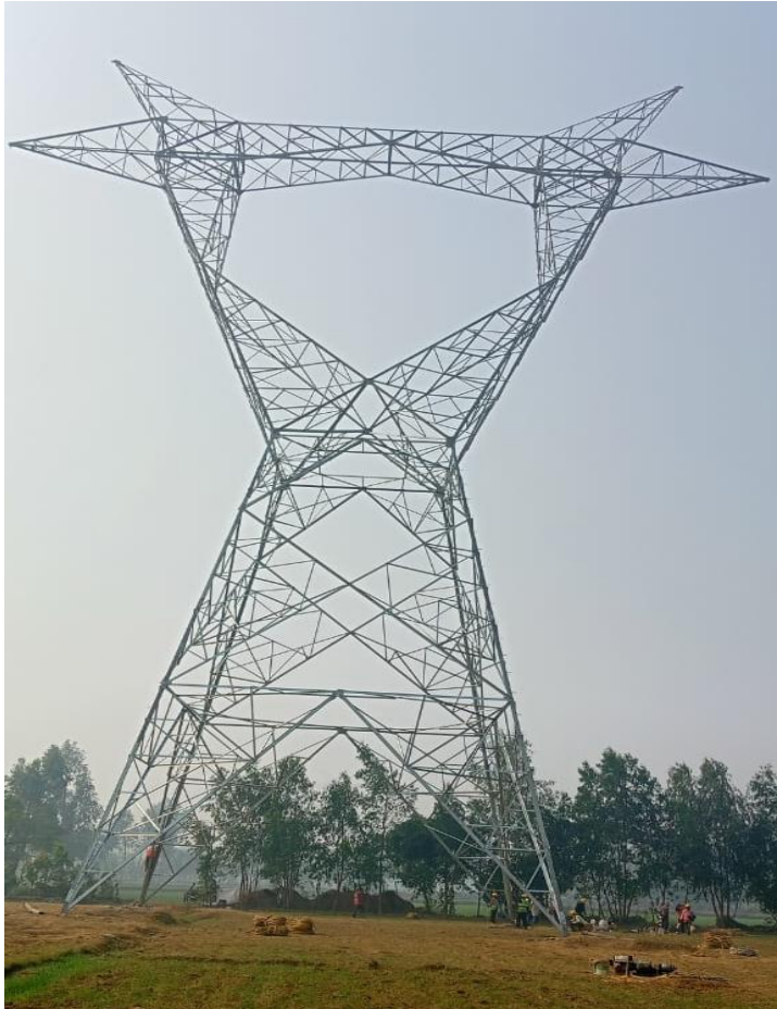
First in house designed 765kV suspension conventional lattice tower, Mohanlal Ganj
