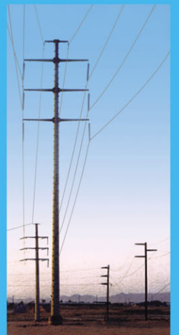
Monopole Transmission Line Tower
