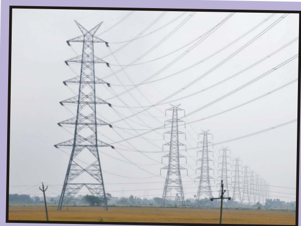
ELECTRIFYING SIGHT: THE 400KV M/C LILO INSTALLATION ON THE NELLORE SRIPERUMBUNDUR LINE AT ALAMATI SUBSTATION.
